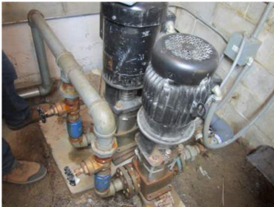
Photo 3: Existing Snowshoe Booster Station Pumps
