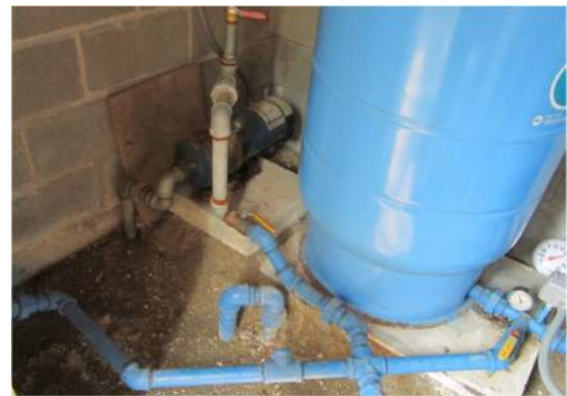
Photo 8: Upper Highland Booster Station
