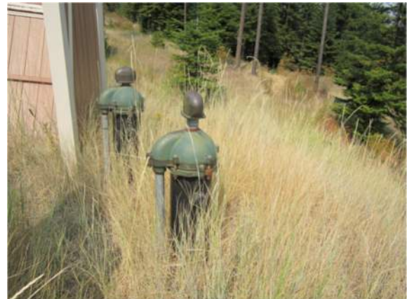
Photo 4: Bella Ridge Boosters Station Pumps
