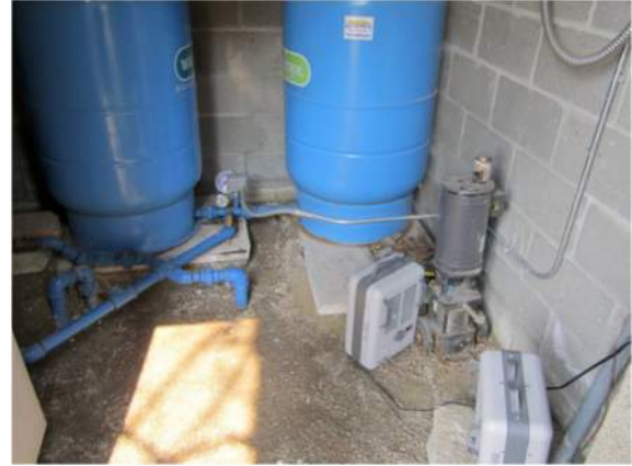
Photo 6: Upper Highland Booster Station Pump and Discharge Appurtenances
