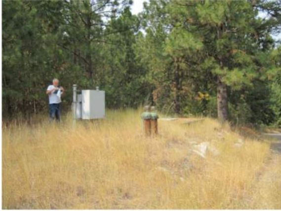
Photo 1: Greenferry Booster Station
