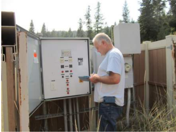
Photo 5: Bella Ridge Booster Station Pump Controls
